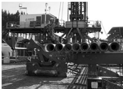
Drill tube for use at Cardiff-3. Image reproduced with permission from TAG Oil Ltd. 2
